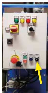
Start/Stop auxiliary pump for particle counter Fig.15
