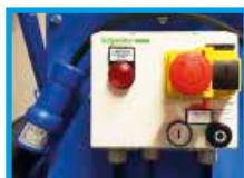
3-phase electrical panel
