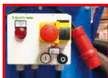
Single-phase electrical panel
